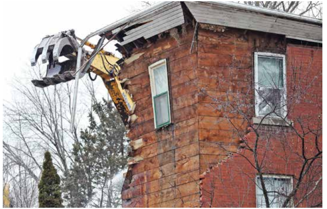
Over 20 long-forgotten interments from the early days of what is now Aurora United Church were found during recent excavations and demolitions of the site.
