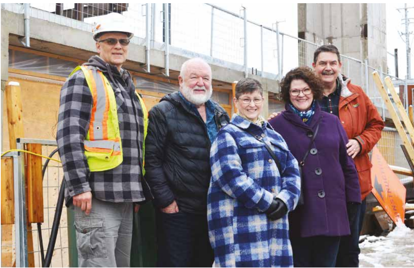
TEN YEARS ON – April 11 marks the 10th anniversary of the fire that devastated Aurora United Church. Last week, as the new church began to take shape at its historic site at Yonge and Tyler Streets, church leaders and parishioners met on site to reflect on the journey. Pictured from left are Construction Manager William Dobson, Brian North, Chair of AUC's rebuilding committee, head of AUC Council Nancy Kerswill, and AUC Reverends Lorraine Newton Comar and Andy Comar. Auroran photo by Brock Weir
